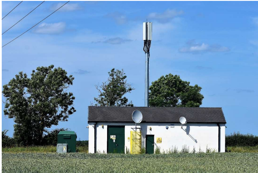
Cellular base station at Langford, and the antenna array
